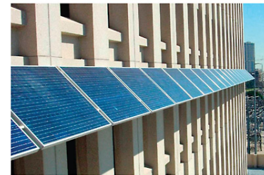
DOE/NREL, University of Texas Health Science Center at Houston AWNINGS
